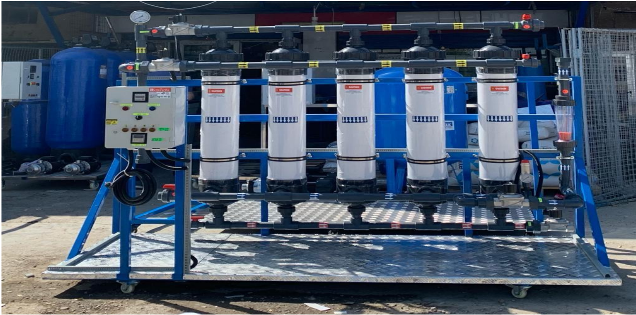
Ultra-Filtration System capacity (15) M 3 /hr.
