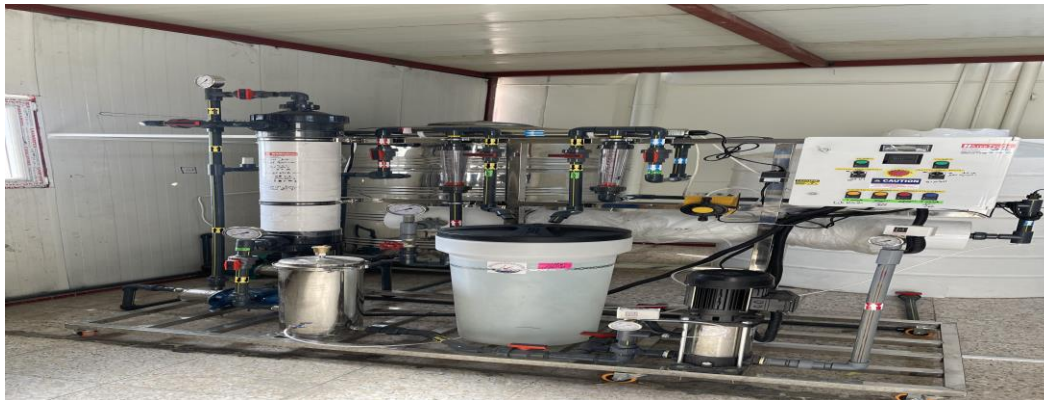
Ultra-Filtration System capacity (4) M 3 /hr.
