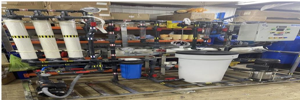
Ultra-Filtration System capacity (2) M 3 /hr.
