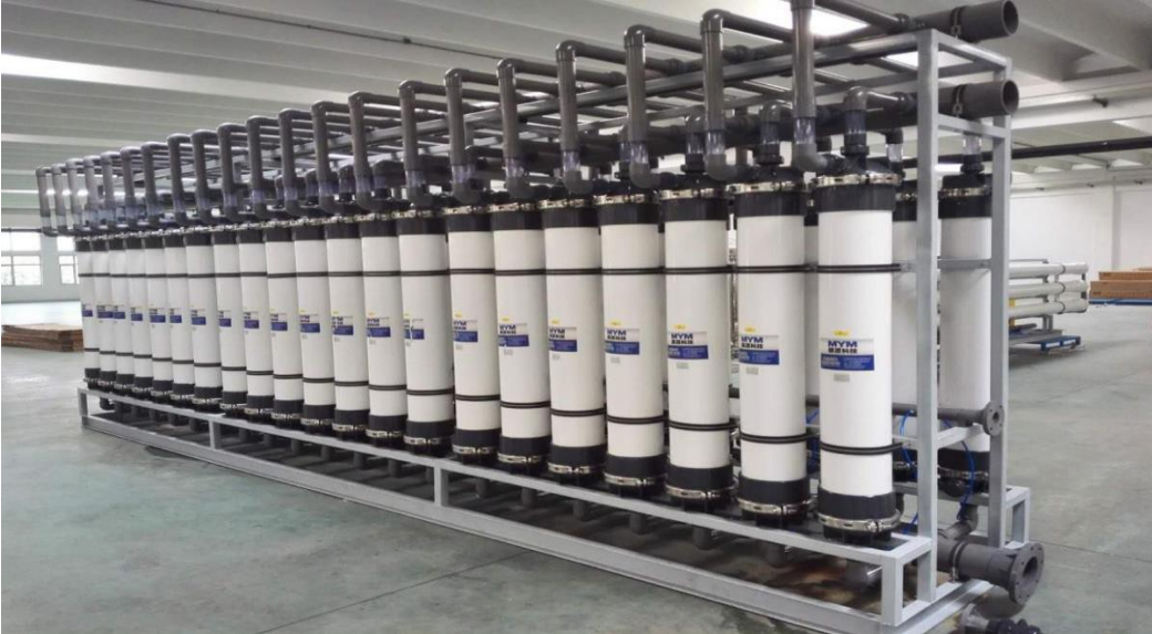
Ultra – Filtration Unit (120) M3/hr.
